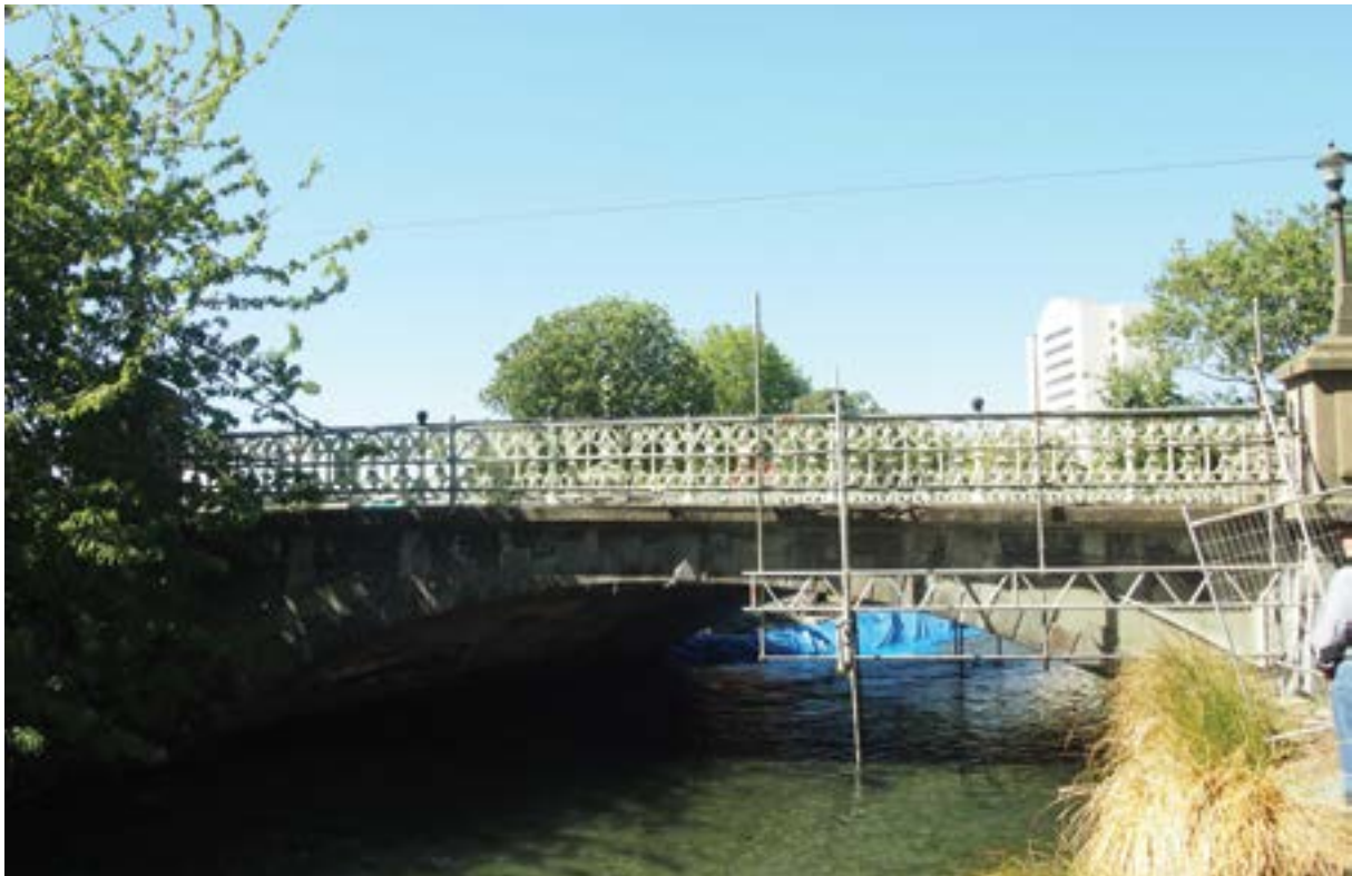
Fig 2. The Armagh Street Bridge, Christchurch, an example of a built structure undergoing work (HNZPT IMG010)
