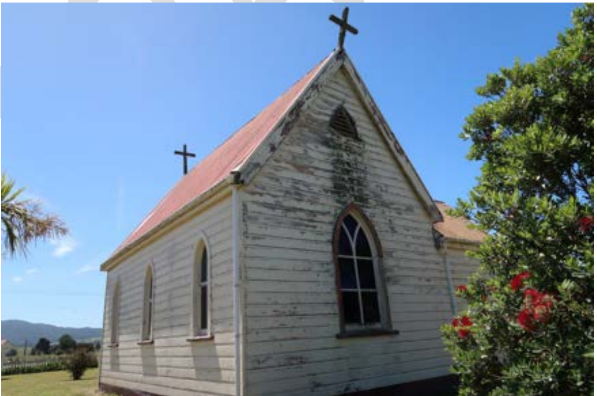
Showing north and west elevations of church with pointed arch windows and tracery, and ventilator in gable
